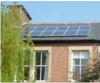
Above, a domestic PV array in Gosforth, with, right, the community orchard in Jesmond
